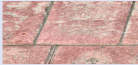
Delaminating sealer can appear as white areas
