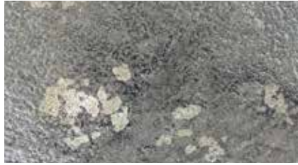
Freeze/thaw cycling and deicing chemicals can cause surface paste to scale or delaminate.
