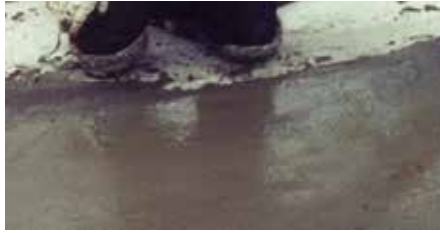
Have realistic expectations about how a functional concrete repair may look.
